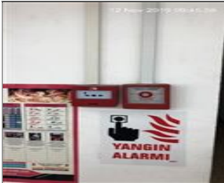
Photo of fire safety equipment firealarm.JPG
