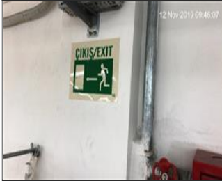
Photo of fire safety equipment exitmark.JPG
